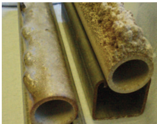
Figure 4 Furnace deposits (RWE npower, 2008)
