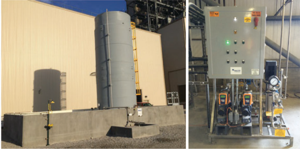
Figure 4 MerControl tank and control system (Maier, 2014)
