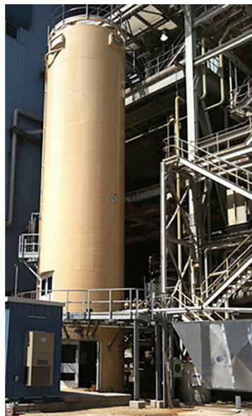
Figure 22 Activated carbon silo (Krents, 2014)
