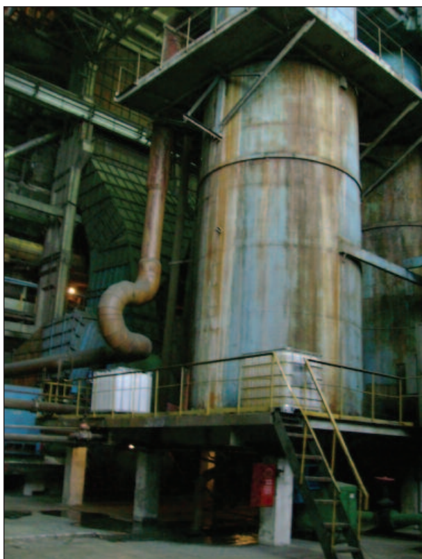
Figure 15 Centrifugal water scrubber at Togliatti Power Plant, Russia (from an as-yet unpublished UNEP report)
