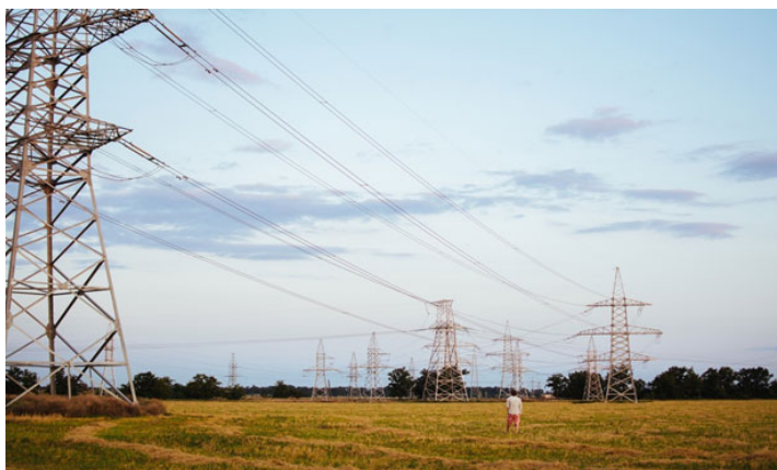
Stock photo of Power Grid in India
