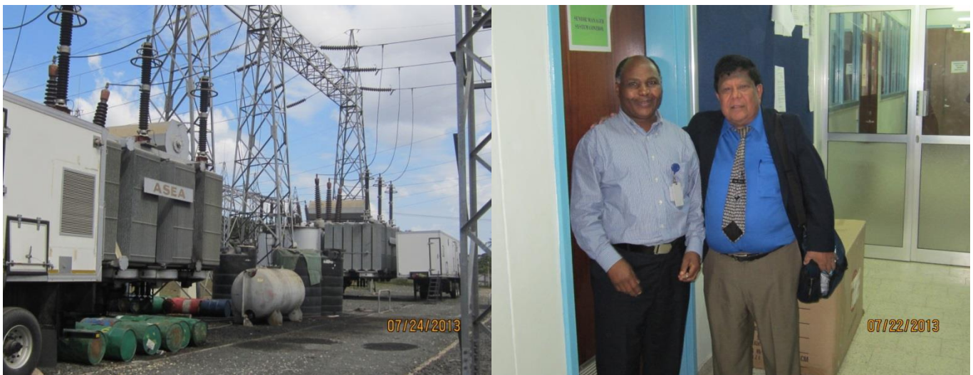
Above left: A 138kV-220kV transformer at TANESCO's Ubungu substation. Above right: USAID/USEA expert Tony Rodrigues meets with TANESCO Manager of Grid Operations Christian Msyani.
