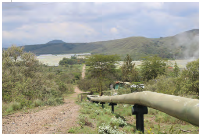
The new geothermal steam supply pipeline will tie in with this existing steam supply pipeline to enable additional power generation from two geothermal power plants.
