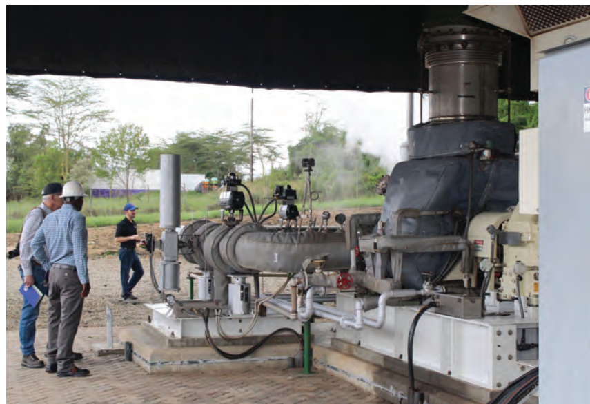
Technical experts examine a 2 MW single-flash geothermal power plant that will provide baseload power to the Oserian Two Lakes Industrial Park.
