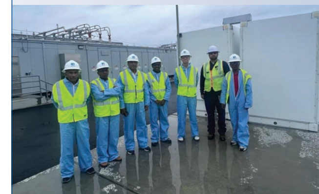
Power sector leaders from Sri Lanka tour Pacific Gas & Electric's Elkhorn BESS site.
