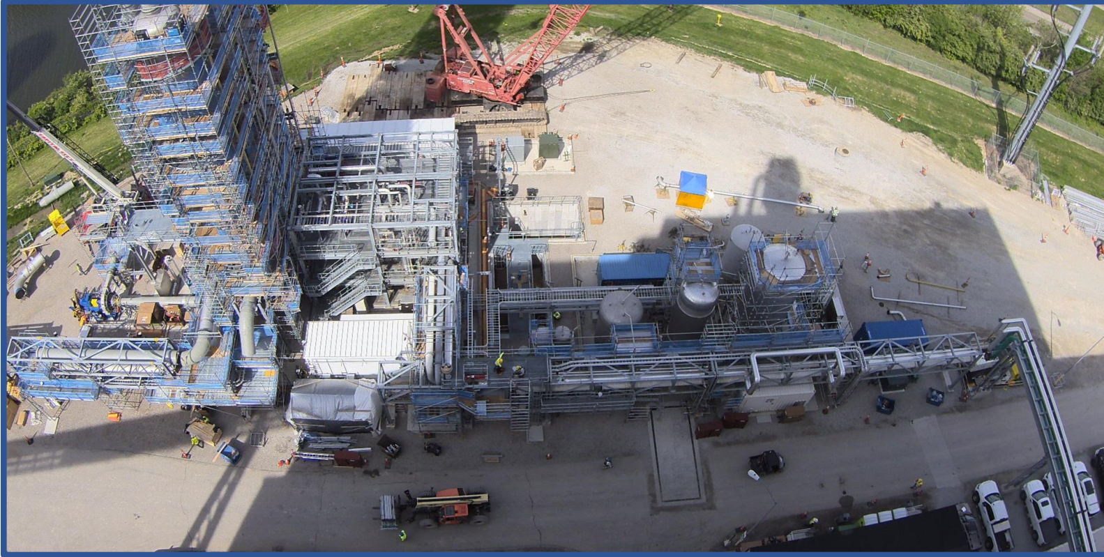
City, Water, Light and Power's (CWLP) Dallman Power Plant
