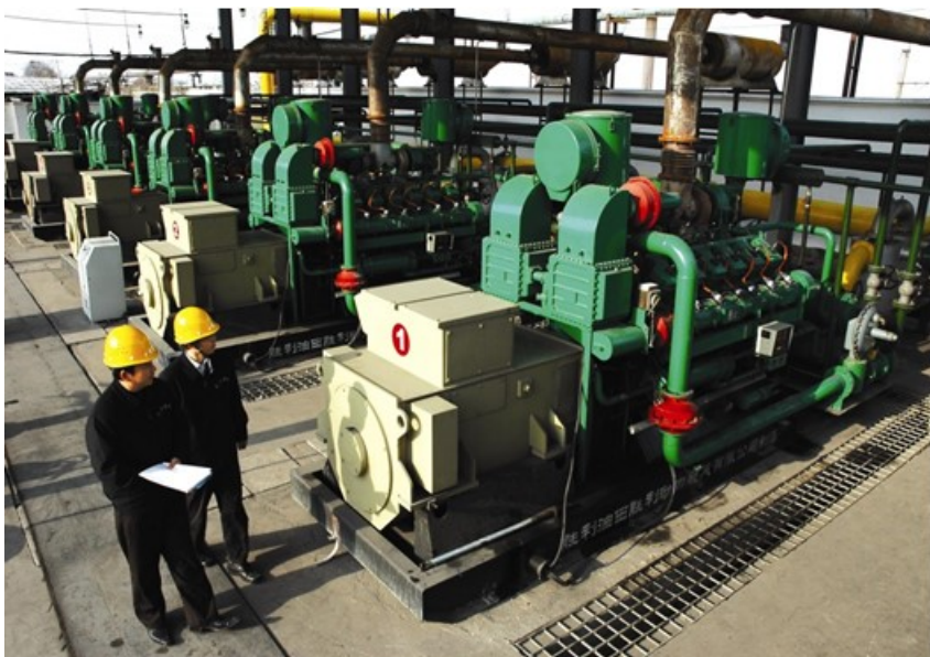
国内外首座6 × 500kw低浓度瓦斯发电站 The first 6 x 500kw low concentration gas power station
