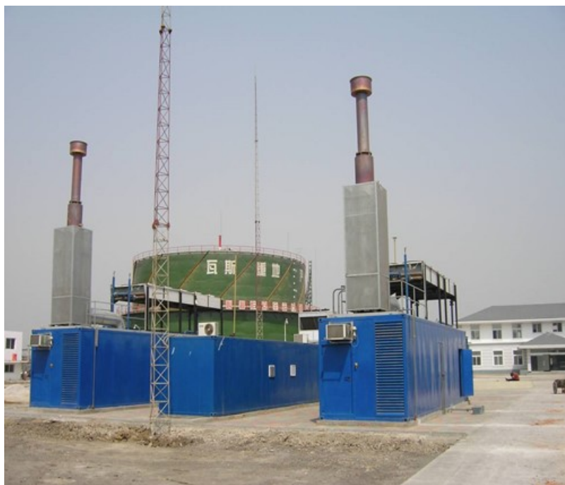
2 × 1360kw瓦斯发电站 2 × 1360kw gas power generation
