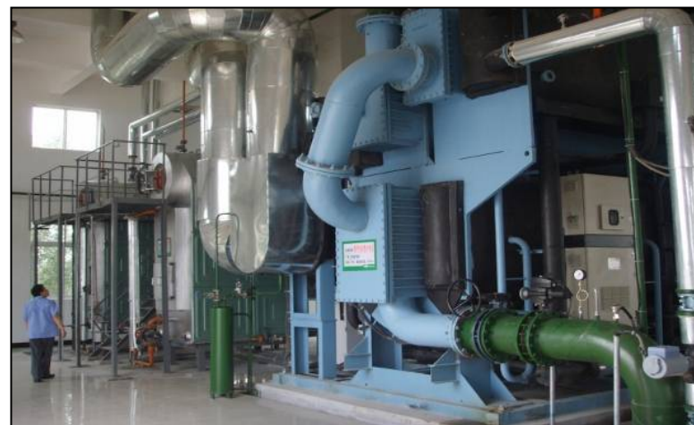
瓦斯发电热电冷联供机组 Equipment of combined cooling, heating and power by gas power generation
