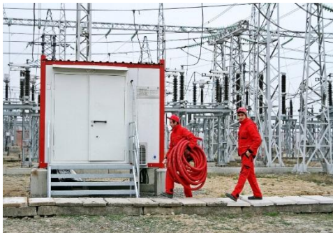
Picture 1 Existing 220 kV Substation Yard
