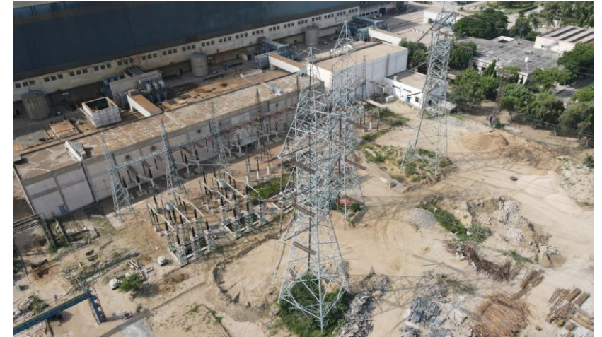
BQPS Transmission Lines
