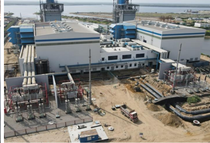
Aerial View of Plant
