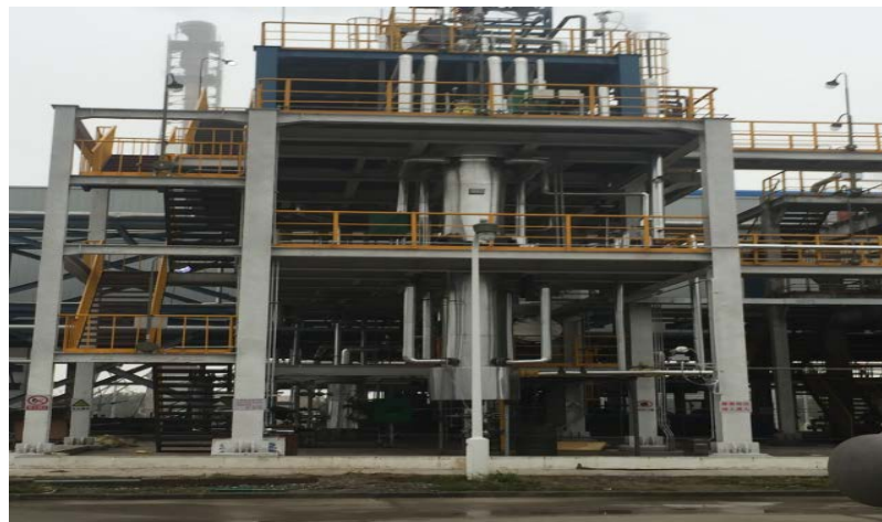
1 kt/a pilot plant test of ethanol synthesis from syngas have conducted in 2016
