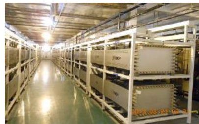
The World Largest Scale System of All Vanadium Flow Storage Battery
