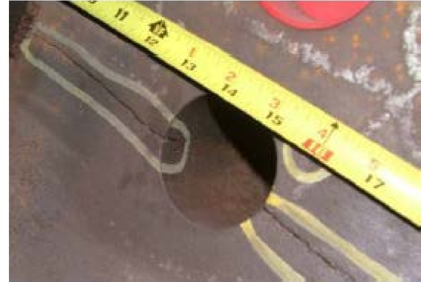
Boiler header ligament cracking due to thermal fatigue
