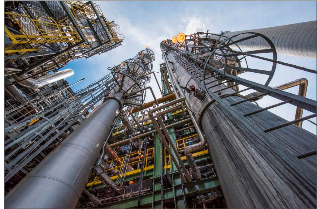
Post Combustion Carbon Capture Center (PC4)
