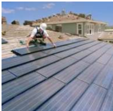
Ladera Ranch, CA 3kW
