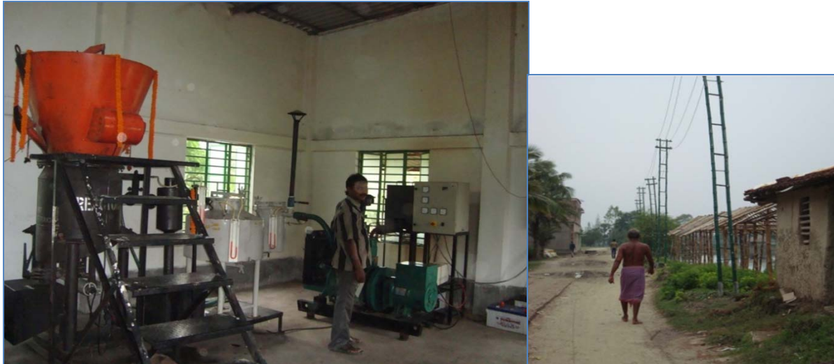
Operational Biomass plant at Sundarbans, West Bengal
